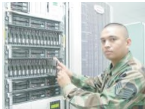
Figure-1-14: SSgt Jay Sablan, AFWA Communications Directorate, Network Systems Administrator, replaces a failed hard drive on an AFWA server.
