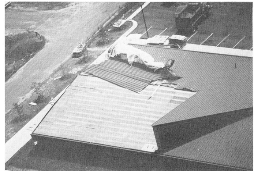
Roof partially blown off of the Arts and Craft Center, Andrews AFB, 1 Aug 83, by a microburst.
